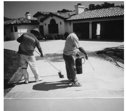
Apply Concrete Colorcoat diluted up to 10% w/water using a airless sprayer or 3/8 - 1/2" paint roller. Apply a topcoat of Sealcoat 1000 clear.
