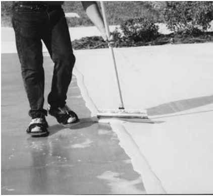
Apply a Squeegee/Bond Coat of Ultra Surface Polymer Concrete over the surface.
